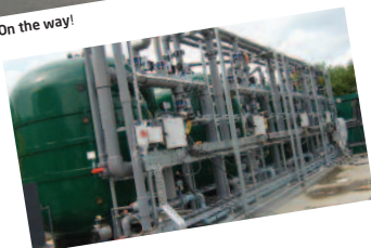
Filters on Site
